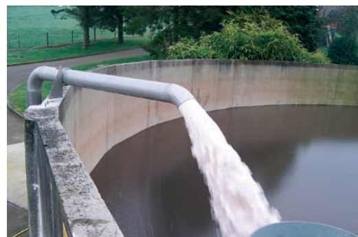
Discharge of Neutralac® SL30 into the tank
