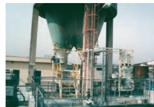
Neutralac ® Duwa-Matic H 2000 positioned under the existing silo
